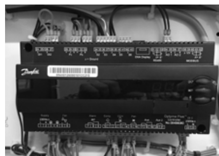
Picture 3: Normal wiring
